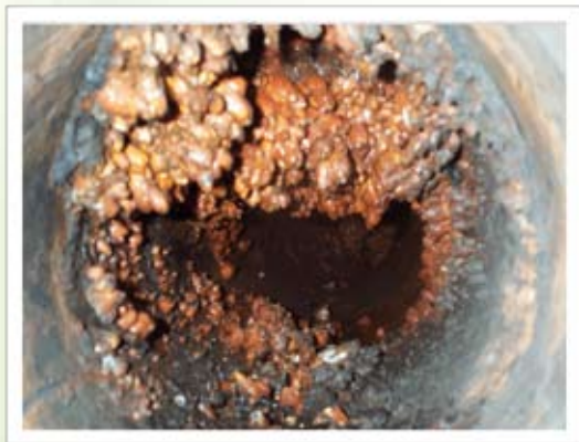
Typical Barnacle Growth in Seawater Piping
